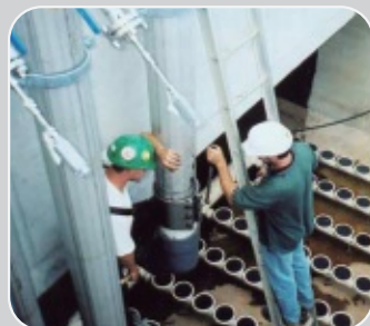
▶ Canada : water puri cation facility
