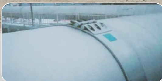
▶ 48 "(1,200A) MF-RL Canadian power plant cooling line
