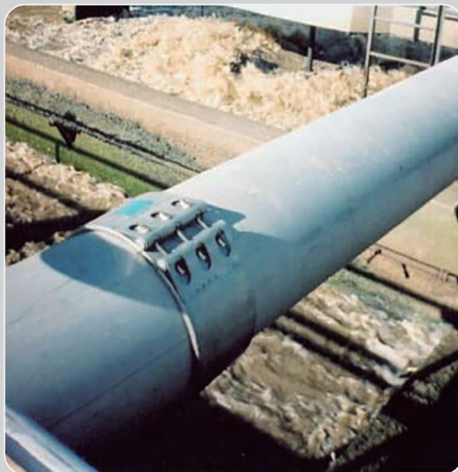
▶ Spain : water puri cation facilities
