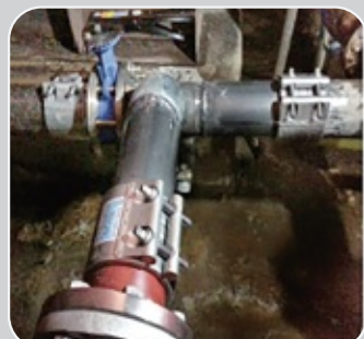
▶ Netherland desalination treatment facilities
