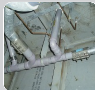
▶ PVC+Steel Pipe Connection
